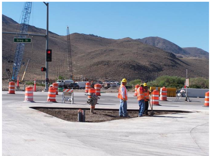
New interchange going in at Greg Street and Sparks Boulevard for the southeast connector roadway
